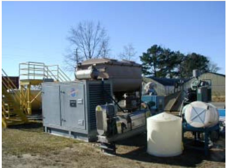
Digester Components Prior to Assembly
